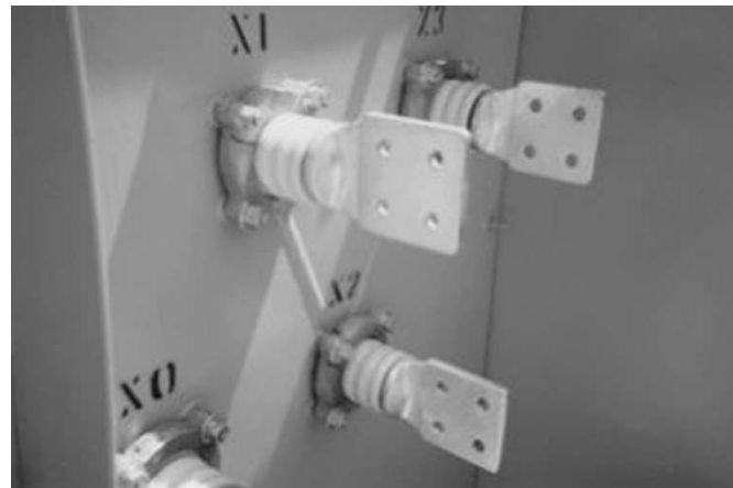
Fig. 10. Transformer with triangular stainless-steel plate on low-voltage side.
